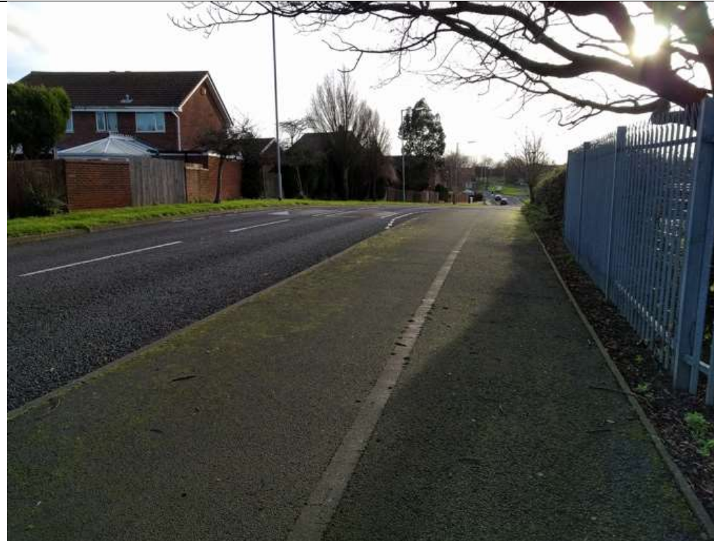
Worn segregated cycle track on Woodland Road
