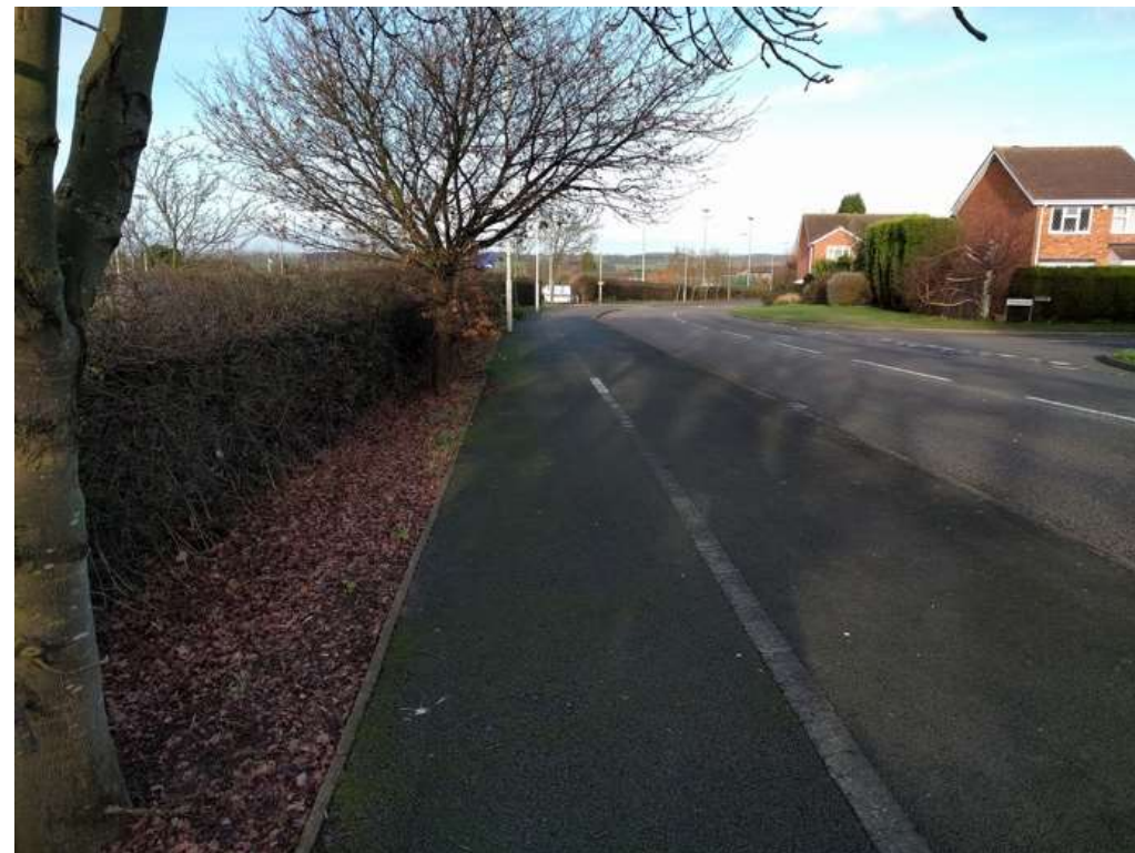
Worn segregated cycle track on Woodland Road
