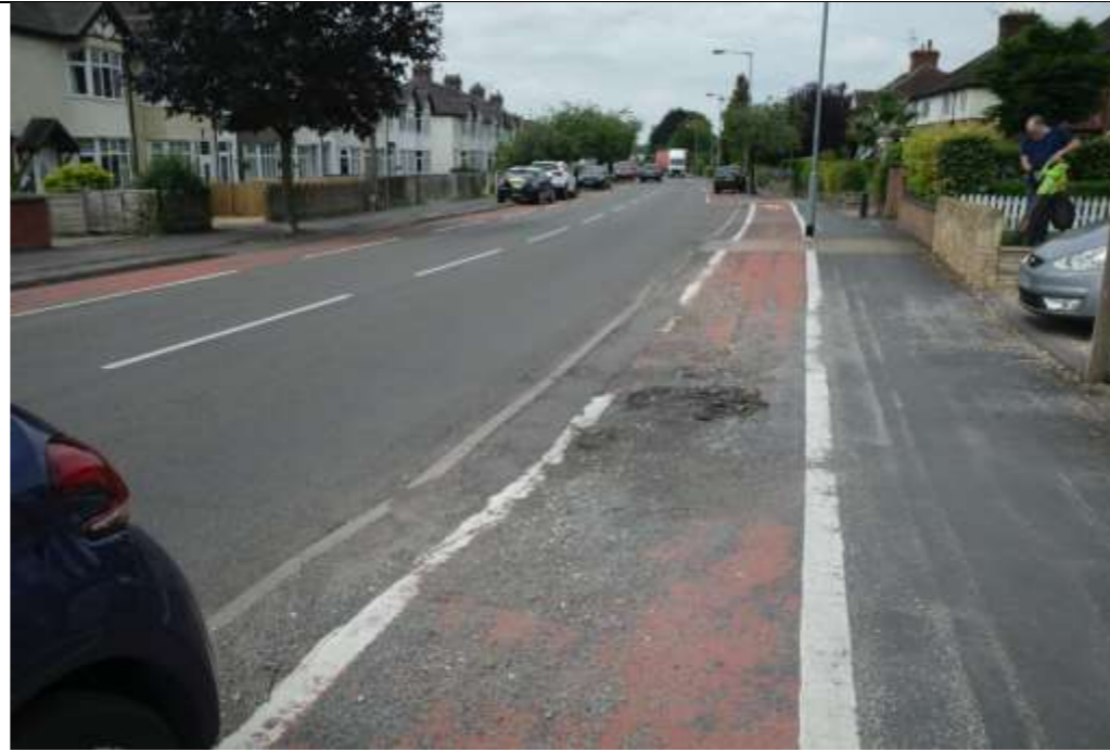
Poor surfacing on segregated cycleway
