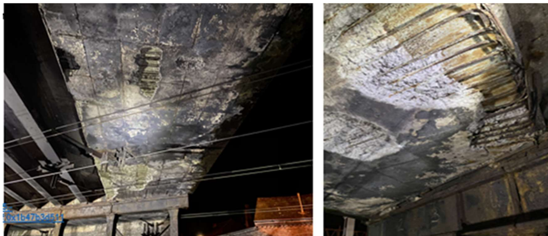
Figure 15 – Stafford Railway Bridge Failure
