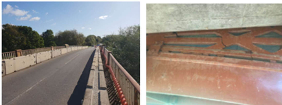
Figure 11 – Chetwynd Bridge Iron Parapet Deterioration
