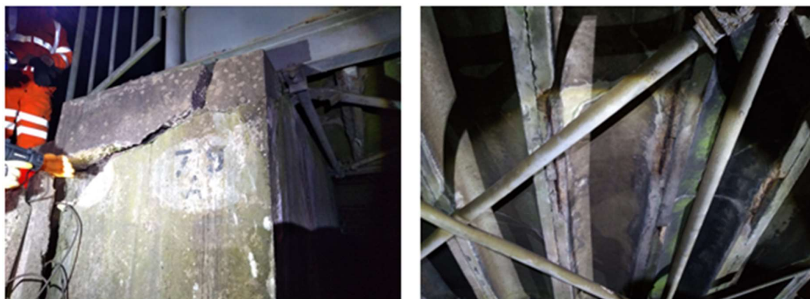
Figure 8 – School Lane Footbridge Deterioration
