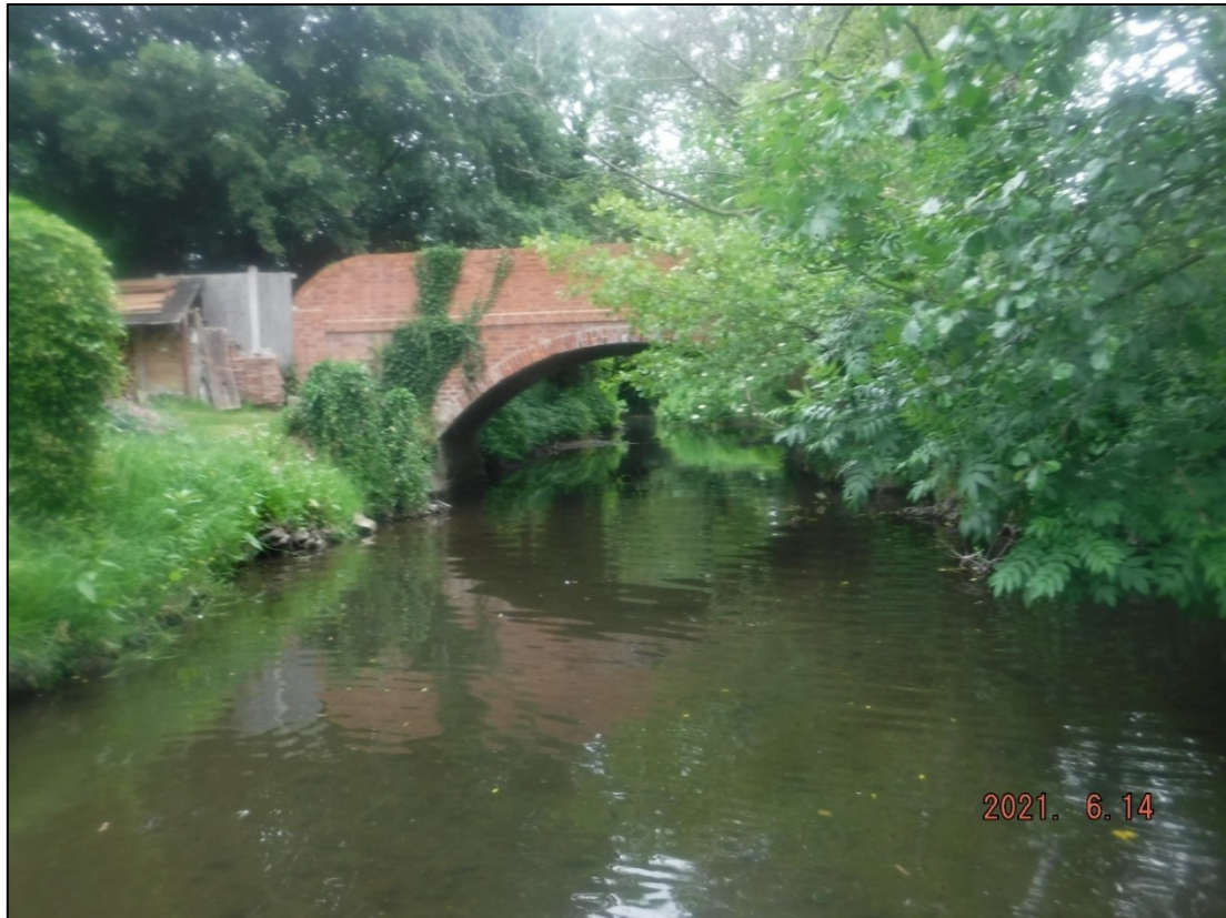
Figure 16: Bond End Footbridge photographed in 2021 during a period of typical flow on the River Swarbour
