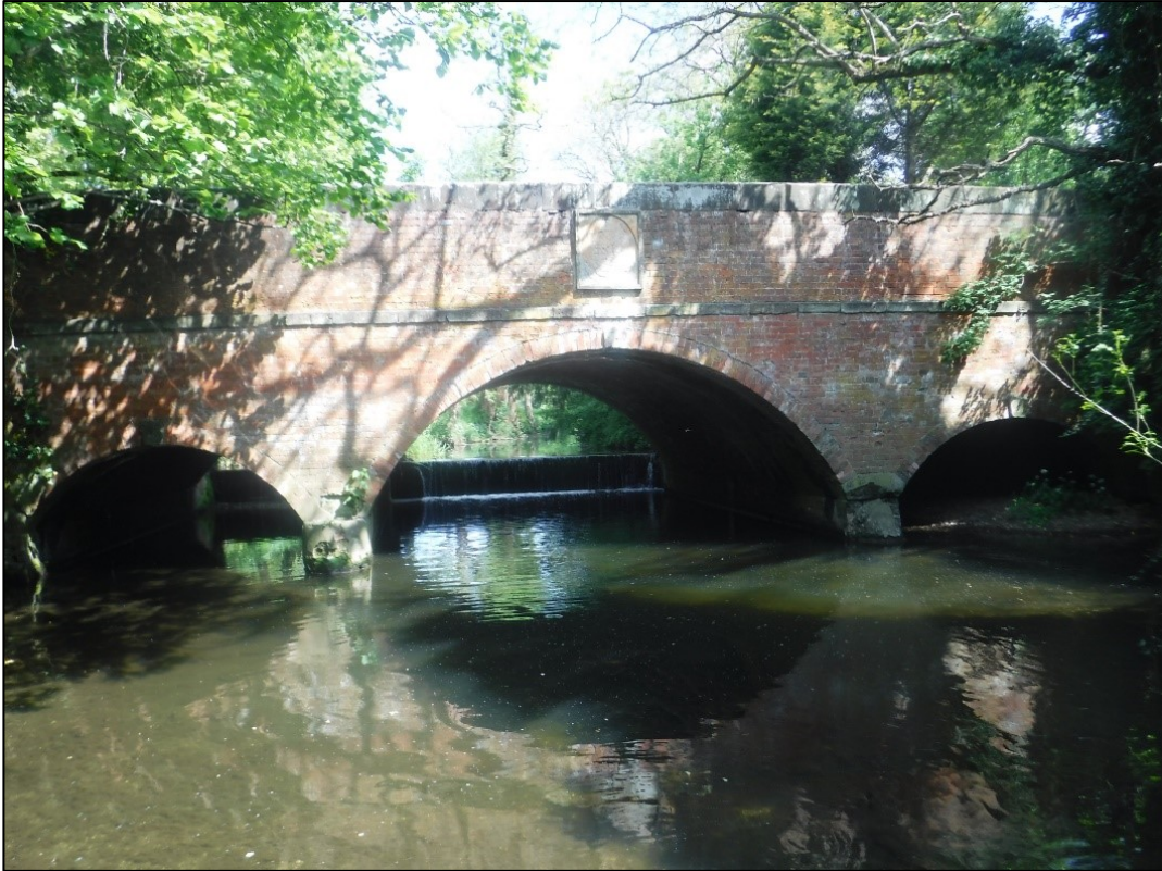
Figure 14: Town Hill Bridge in May 2019 showing no blockage prior to February 2020 Flood Event
