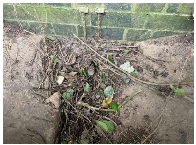
Figure 16: Culvert A outlet pipe from field with blockage to pipe as observed on site in March 2022
