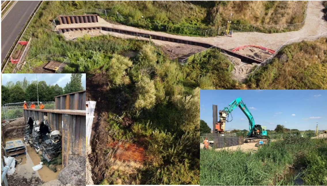
Figure 16: Construction of the scheme in area one, the low spot on the east of the Lichfield Road highway (image source and rights belong to the Environment Agency)
