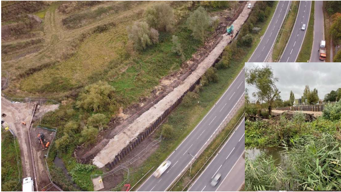
Figure 18: Construction of the scheme in area three, alongside the east of the Lichfield Road/A38 (image source and rights belong to the Environment Agency)
