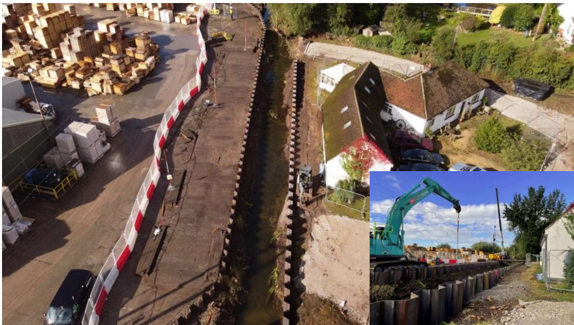
Figure 17: Construction of the scheme in area two, alongside the Tatenhill Brook (image source and rights belong to the Environment Agency)
