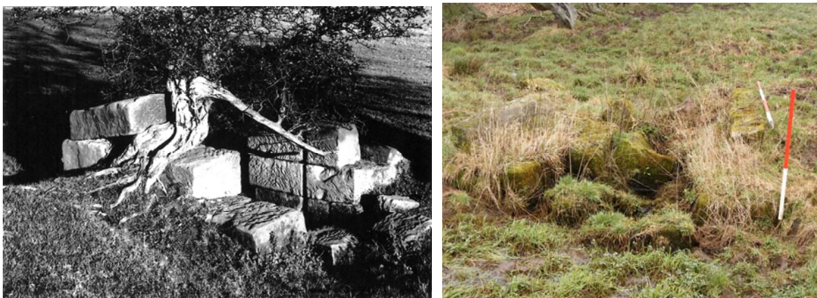
Figure 61- Damage to former sluice structure over time, Willows Farm
