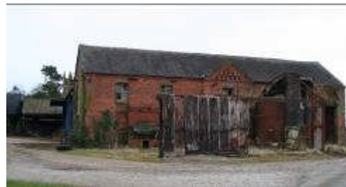
Figures 7 and 8 Two sides of a small L-plan range in west Staffordshire with numerous openings to both elevations of the main range
