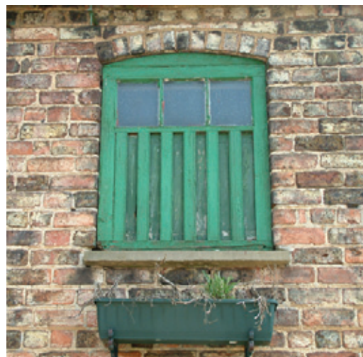
Hit and miss ventilator. Photo © Jeremy Lake
