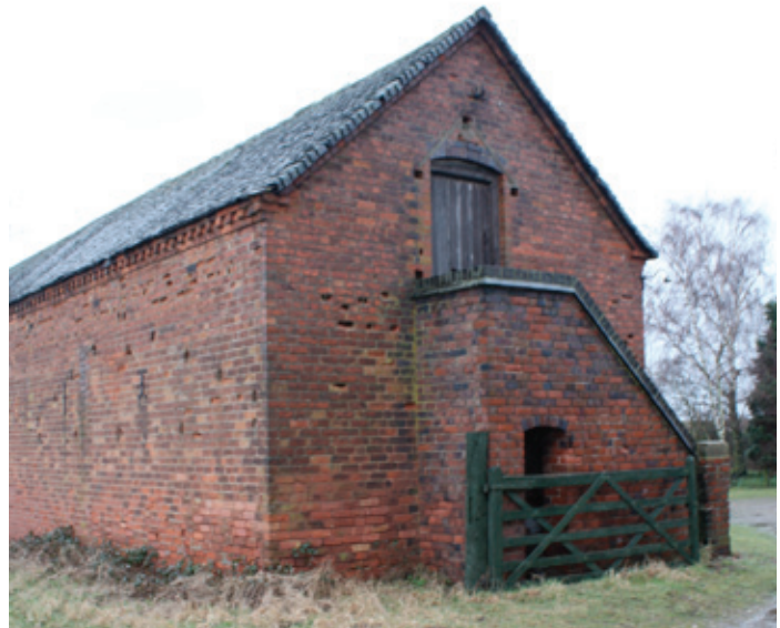
Kennel set in a recess under granary steps, Trent Valley. Photo © Bob Edwards
