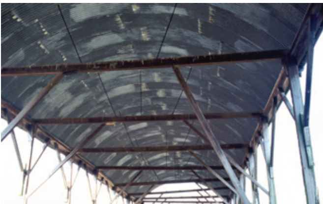
Late 19th century Dutch barns built partly of timber can have wrought-iron struts to a corrugated iron roof and cast-iron braces to strengthen the construction. Photo © Joan Grundy
