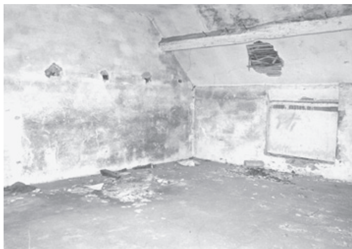
Plaster floor and walls to a cheese room at Birchensale Farm, Redditch. Photo © Worcestershire County Council
