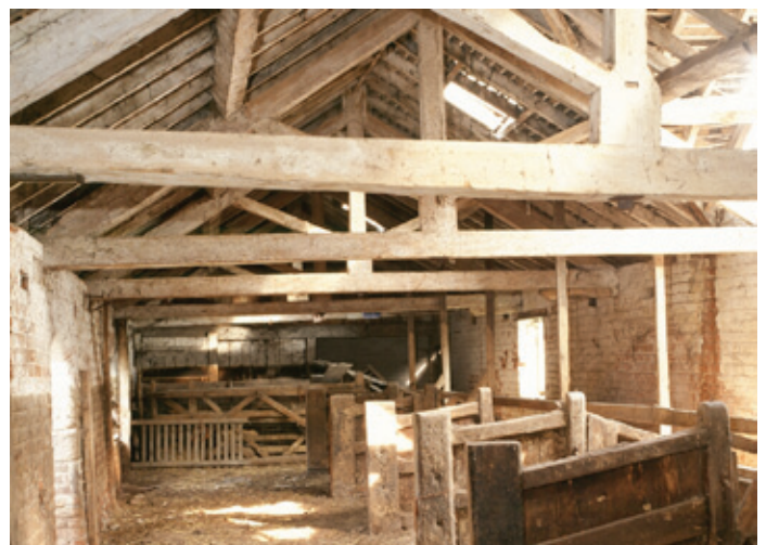
Interior of a cow house showing wooden stalls and king post roof. King post roofs made from imported softwood with iron stays and bolts comprise a standard form of roof truss used in the 19th century, most commonly from the 1840s. Photo (c) Mike Williams/ English Heritage
