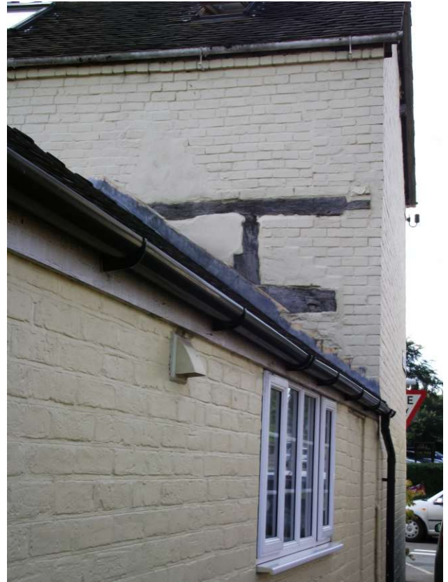
Plate 14: Timber frame in rear of 7 Horsefair
