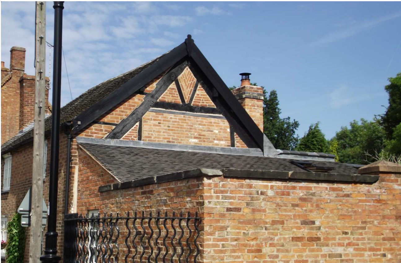
Plate 12: Evidence of earlier timber framed origins in the gable end of a listed property on Bagot Street
